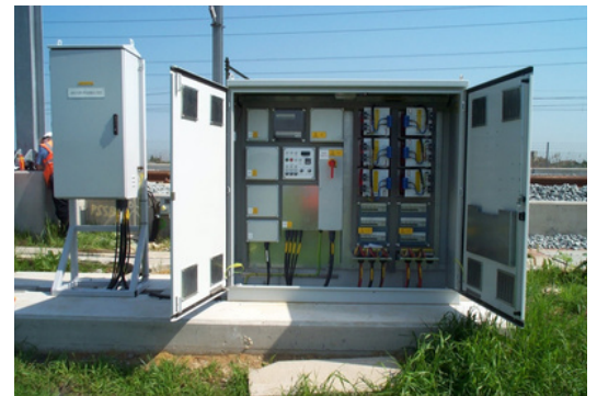
6 Transformer Cubicle with Site Lighting Enclosure
