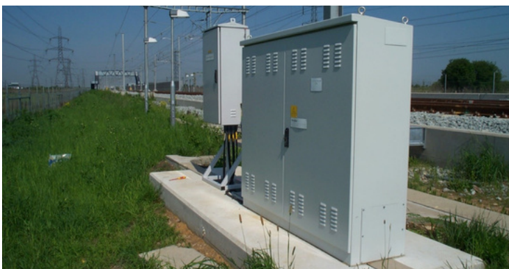
6 Transformer Cubicle with Site Lighting Enclosure
