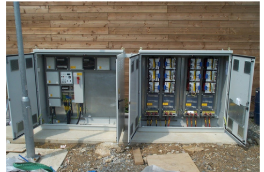
12 Transformer Control & Transformer Cubicle
