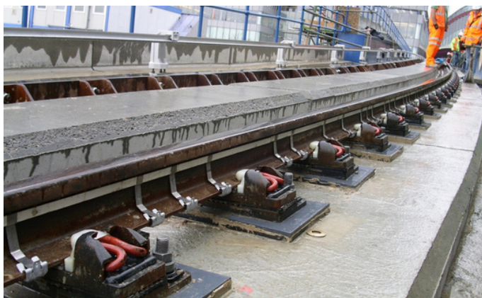
West India Quay 22m Heater Strip
